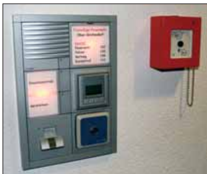
Picture 2. Thanks to the integration of different trades, the doors open and the lights are switched on by the fingerprint terminal of the access control system.
