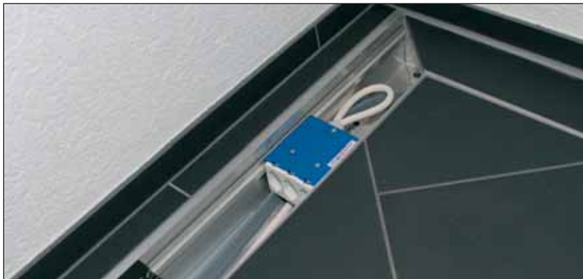
Figure 2. Floor conduits allow later retrofits
