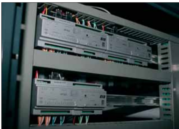
Figure 3. The KNX audio components allow the access of different sound sources from every room and the control of the sound and volume
