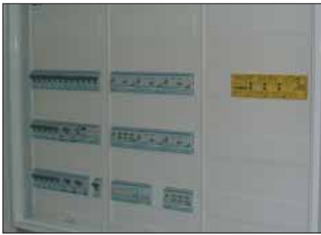
Figure 2. KNX components of the central apartment distribution
