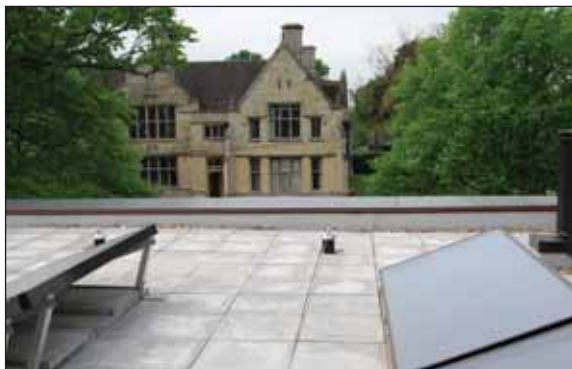
Picture 3. Sustainable Energy Sources: Solar collectors for domestic water heating.
