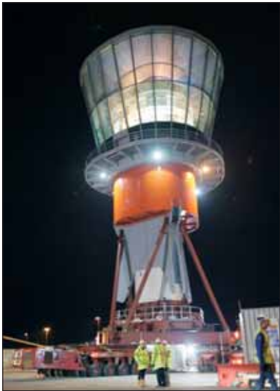
Figure 3. Parts of the control tower on its way to the project site
